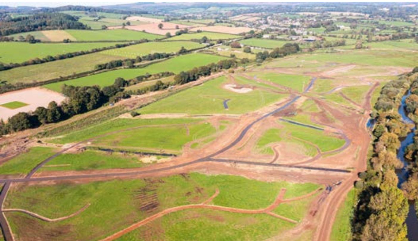
© Clinton Devon Estates: New creek and flood plain channels connecting to the historic river Otter floodplain
